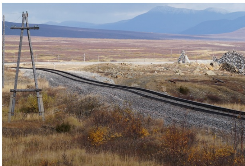
Figure 1: Differential Thaw Settlement of Railways on Permafrost Terrain
